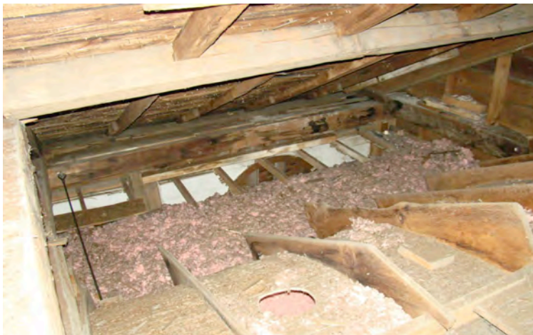
Looking down from 1811 ceiling height showing framing for recessed cove and arch top to 1811 windows still in place.
