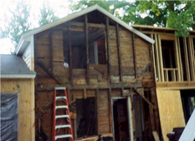
Circa 1815 timber frame, gable end with braces, second story floor cross beam and no cross beam at roof plate.
