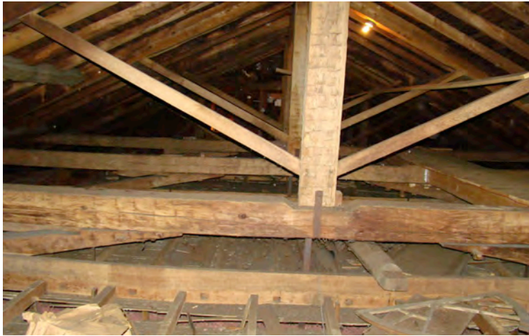
Timber frame at peak in attic with later alterations to ceiling framing, 1867.
